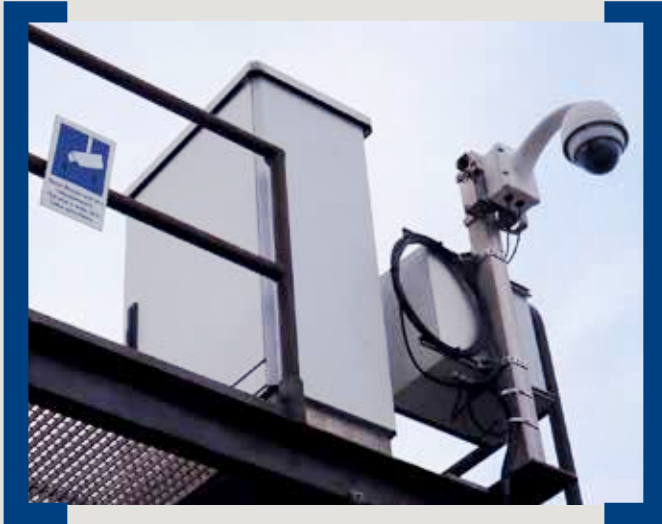
Compliance with data protection regulations in the use of CCTV systems
