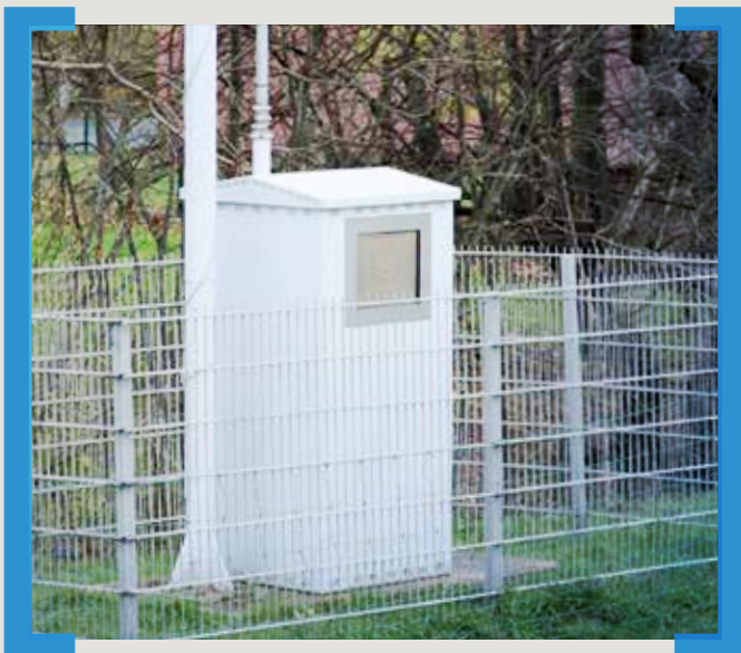
Noise monitoring station in Weddewarden
