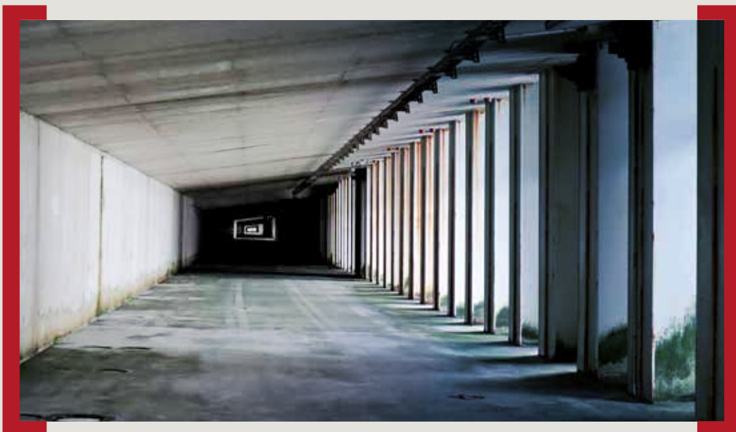
The wave absorber underneath the Container Terminal is part of our coastal protection infrastructure
