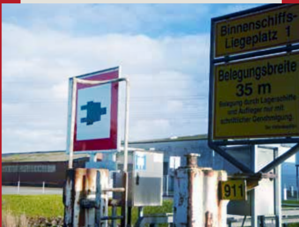
Inland shipping berth with shore power connection at Bremen's Industriehafen
